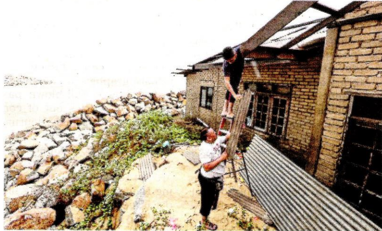
Yushrey A. Rashid, (left) and his brother-in-law, Mohd Nazrin Mohd Yahya (on the ladder), repairing the roof of their house that was damaged by the tropical storm Pabuk in Kuala Nerus yesterday. PIC BY GHAZALI KORI
